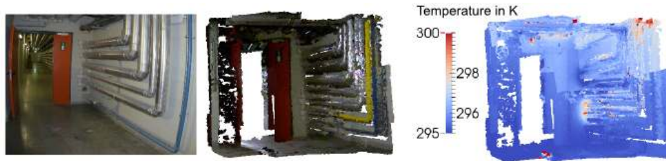
Figure 12. Second 3D-representation of a utility corridor 2. Left: Picture of the place. Middle: Visual-3D representation. Right: Thermal-3D representation.
