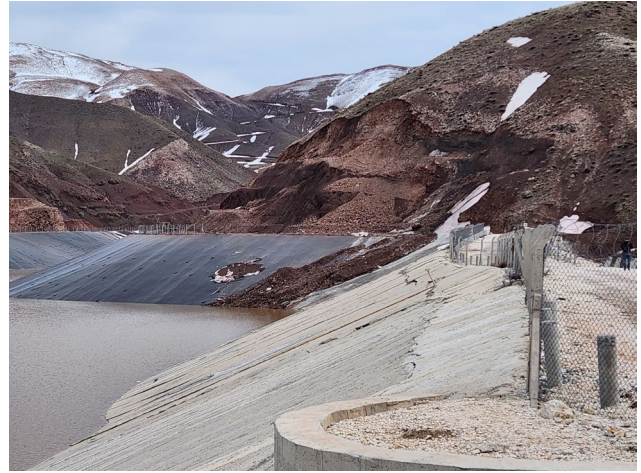
Figure 9. A view from the Erkenek dam body cut by the surface rupture
