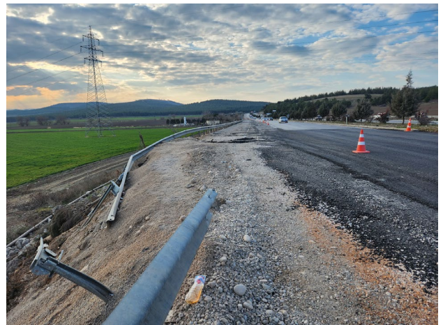
Figure 6. The Gaziantep – Kahramanmaraş State Rod cut by the surface rupture
