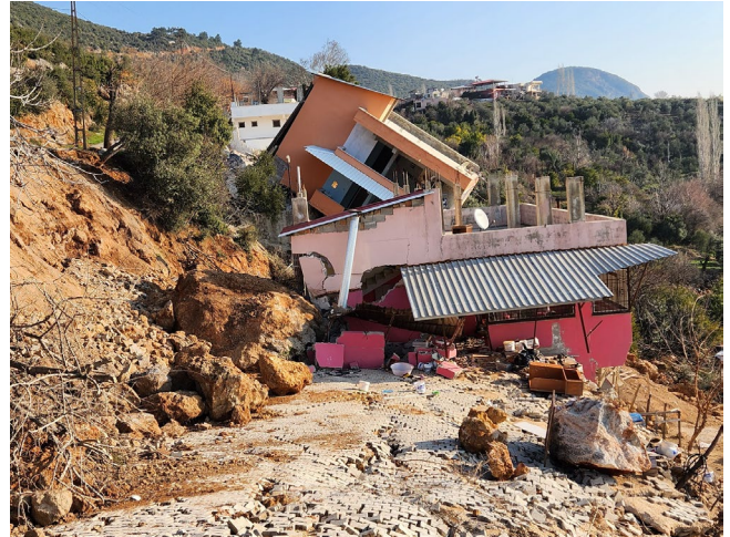
Figure 18. A view from the rockfalls in Bektaşlı village, Kırıkhan
