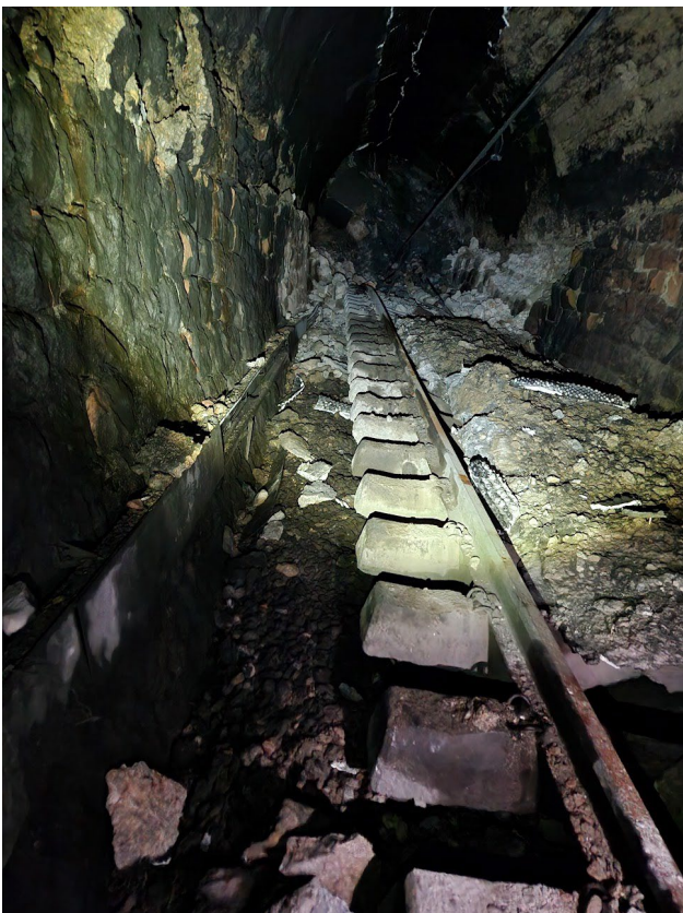
Figure 8. A view from the collapsed T3 tunnel
