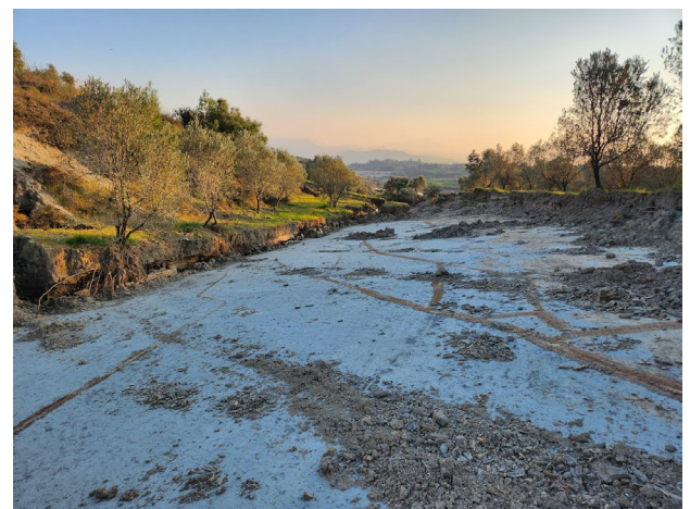
Figure 14. A view from the failure surface of the planar failure
