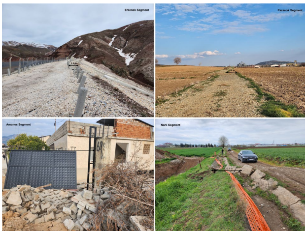
Figure 4. Some views from the left lateral displacements occurred during the Pazarcık Earthquake.
