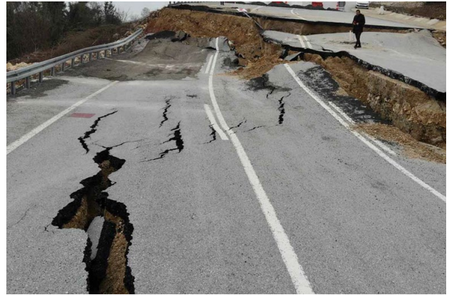
Figure 5. The TAG Motorway cut by the surface rupture (TRT Haber, 2023)
