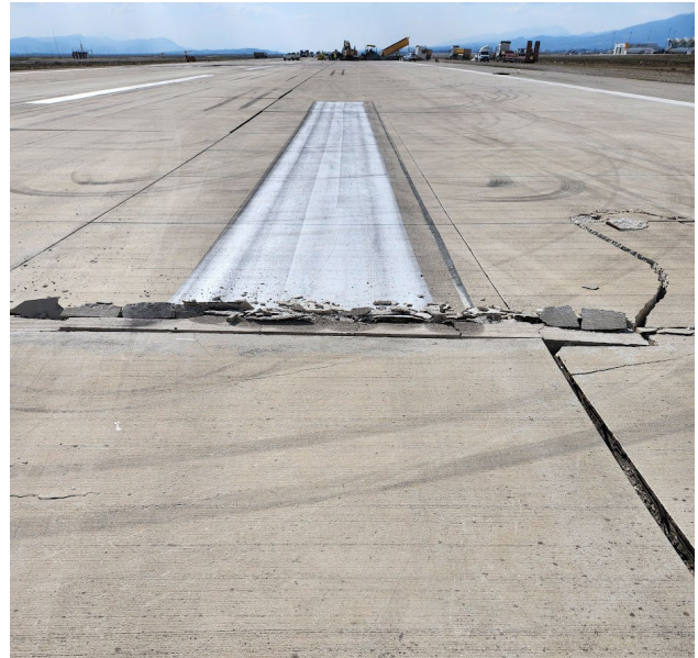
Figure 26. A view from the runway damages of the Hatay Airport
