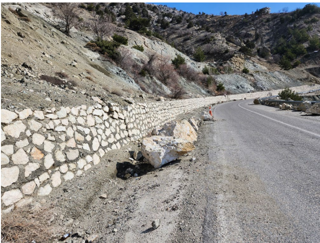
Figure 16. A view from the rockfall on the Gölbaşı – Nurhak road
