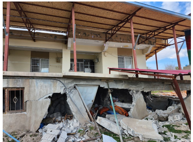
Figure 10. A view from a double stories building cut by the surface rupture (Tetirlik village, Pazarcık)
