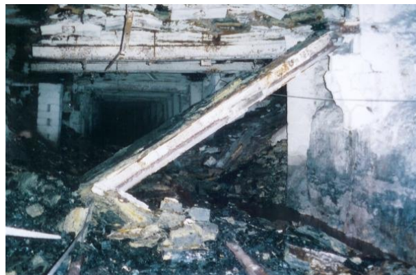
Fig. 7. Fallen roof timber 308 meters inside portal 1 (Photograph Courtesy PA-DEP)
