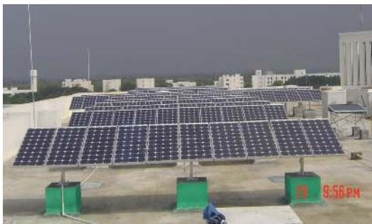
FIGURE 13: 10kW SPVA (14 × 10) installed in open terrace of EEE department block by SSNRC (BELL Laboratories).
