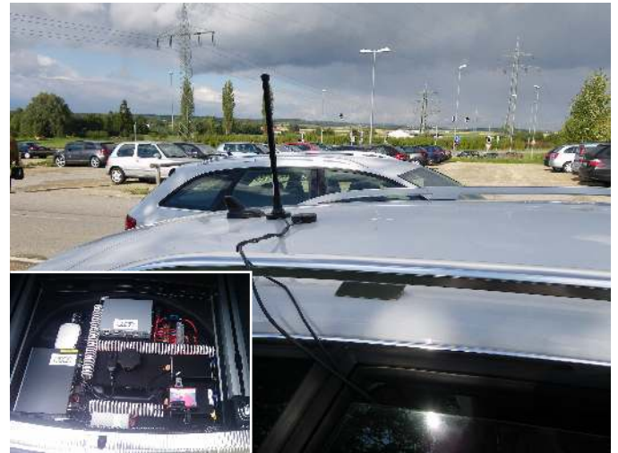
Fig. 2: Position of the shark fin antenna assembly, omnidirectional antenna, and GPS receiver on the roof; installation of the DENSO WSU 802.11p radio in the trunk (inset).
