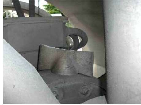
FIGURE 3: An example of a fan blade with a blade mechanical failure at the root aerofoil interface. This fan operated for approximately ten hours in a stalled condition before the mechanical failure [46].
