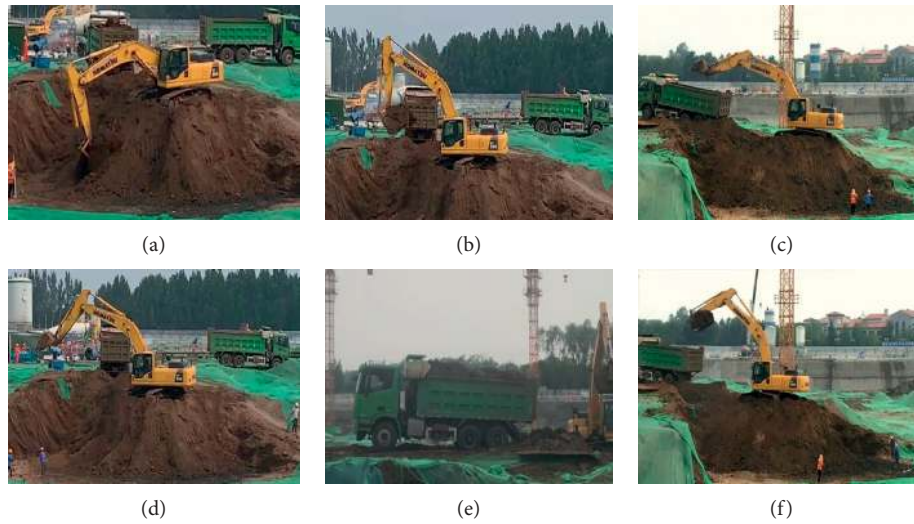
FIGURE 1: Examples of the activities of an excavator and a dump truck: (a) excavator digging, (b) excavator swinging, (c) excavator dumping, (d) excavator swinging, (e) dump truck moving forward, and (f) dump truck moving backward.
