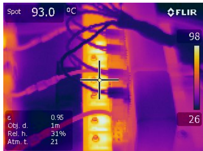
Fig. 23. Thermal image of the switching devices under fan assisted normal operation
