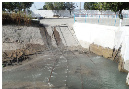
Fig. 6. Testing of a device to reduce siltation of the front chamber of the pumping station «Sputnik».
