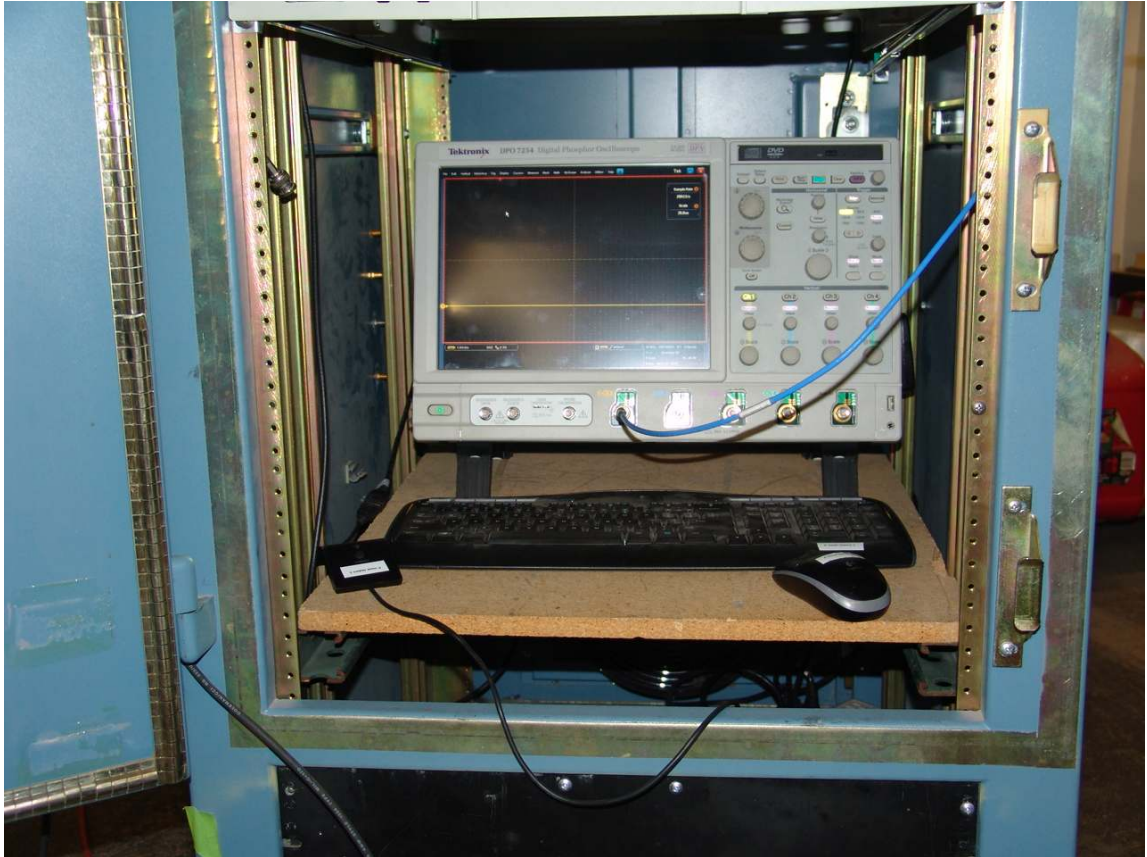
Figure 79. Tek. DPO 7254 Oscilloscope in Screened Enclosure
