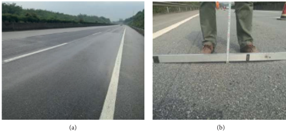
FIGURE 7: Rutting of Guangyun Expressway.
