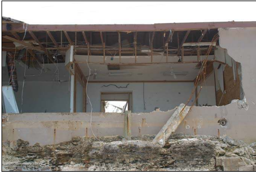
Picture B.26 – Hurricane Jeanne Damage on the Island of Abaco, The Bahamas (Source: NEMA, 2004)
