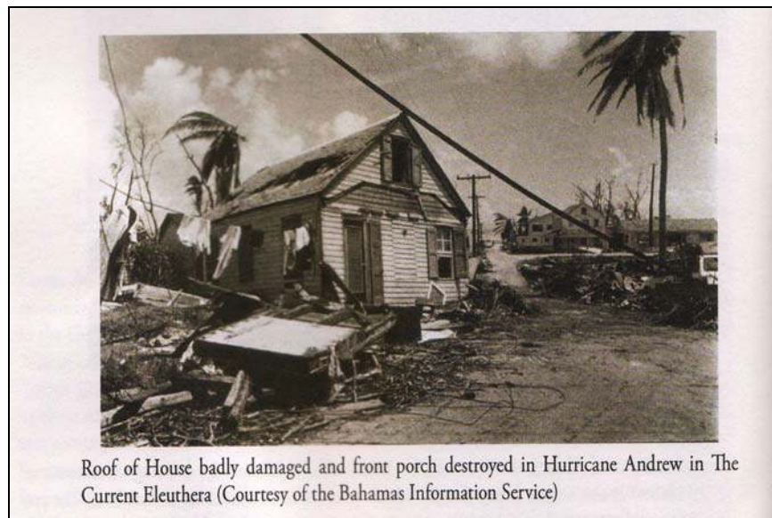
Picture B.3 – Hurricane Andrew Damage on the Island of Eleuthera. (Source: The Bahamas Information Service published in Neely 2006)
