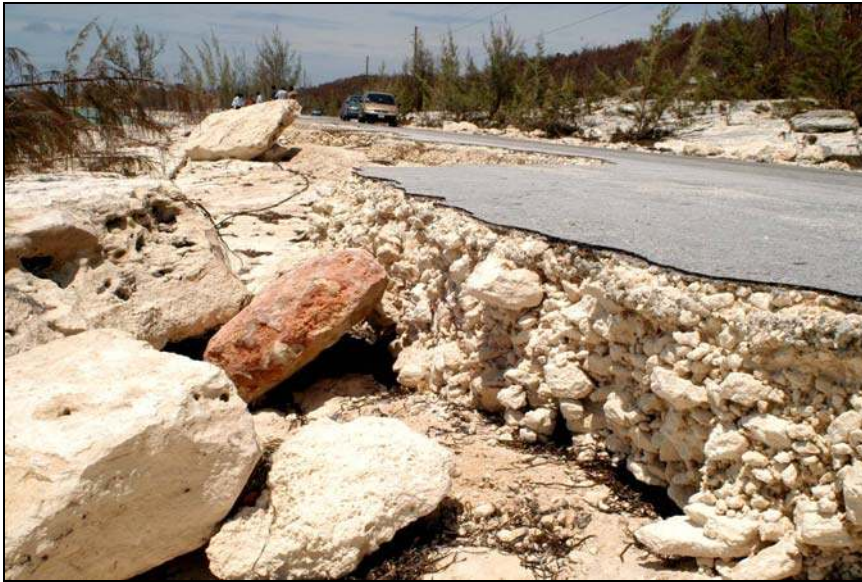
Picture B.19 – Hurricane Frances Damage in the settlement of Gregory Town on the Island of Eleuthera, The Bahamas (Source: NEMA, 2004)
