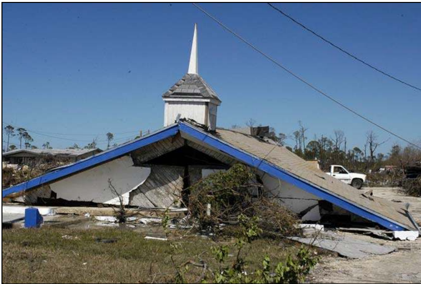
Picture B.36 – Hurricane Wilma Damage. Ray of Hope Church, Hanna Hill, Grand Bahama (Source: NEMA, 2004)
