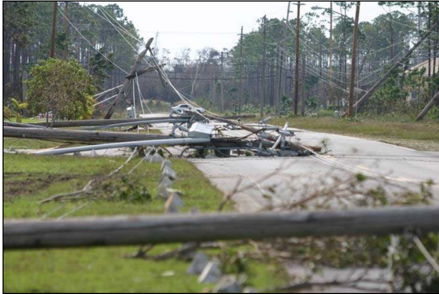
Picture B.17 – Hurricane Frances Damage on the Island of Grand Bahama, The Bahamas (Source: NEMA, 2004)
