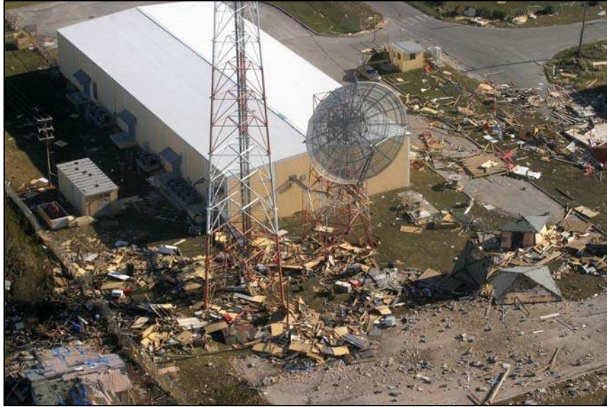
Picture B.35 – Bahamas Telecommunications Company Building Hurricane Wilma Damage, Jones Town, Grand Bahama (Source: NEMA, 2004)
