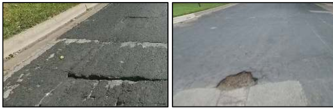
Fig. 7. Instances of road anomalies: deep transverse crack and pothole.
