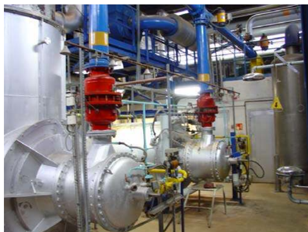
Fig. 2. An inside view of the incinerator hall at DSM Resins. The photograph is taken from the position corresponding to the lower left corner of Fig. 1, showing the cyclone next to antenna position 5 at the rightmost of the picture.
