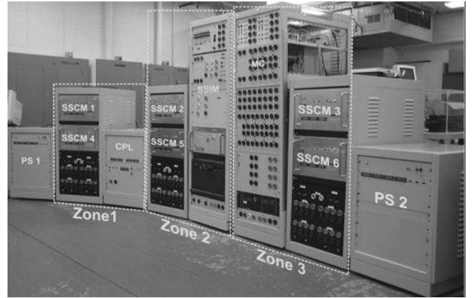
Fig. 2. Hardware of the dc distribution testbed.
