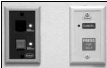
Image 5 (b)_Light switchboards in the phlebotomy drawing room used for communication with the master control board.
