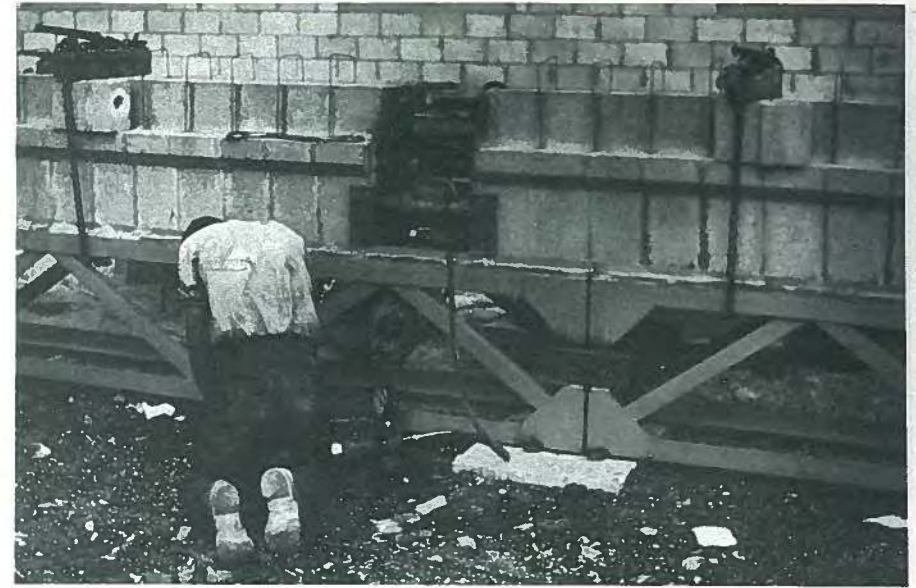
Fig. 10. Tensioning two 16x24-in. (406 x 610 mm) block building beams by jacking them apart.
