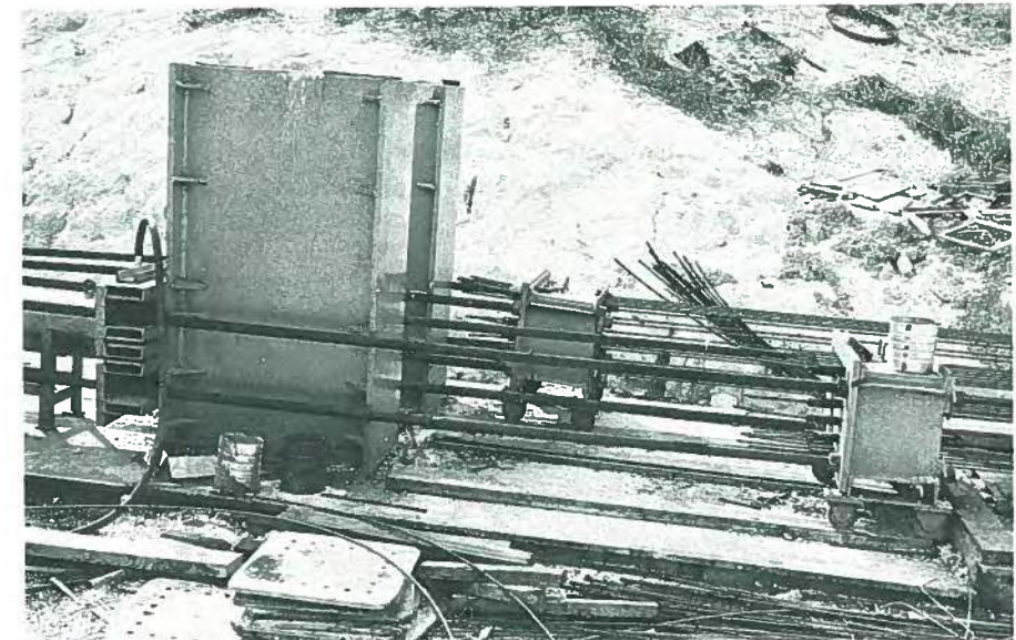
Fig. 33. Early multi-strand tensioning of an 18-in. (457 mm) square pile. Courtesy: Dura-Stress, Inc., Leesburg, Florida.
