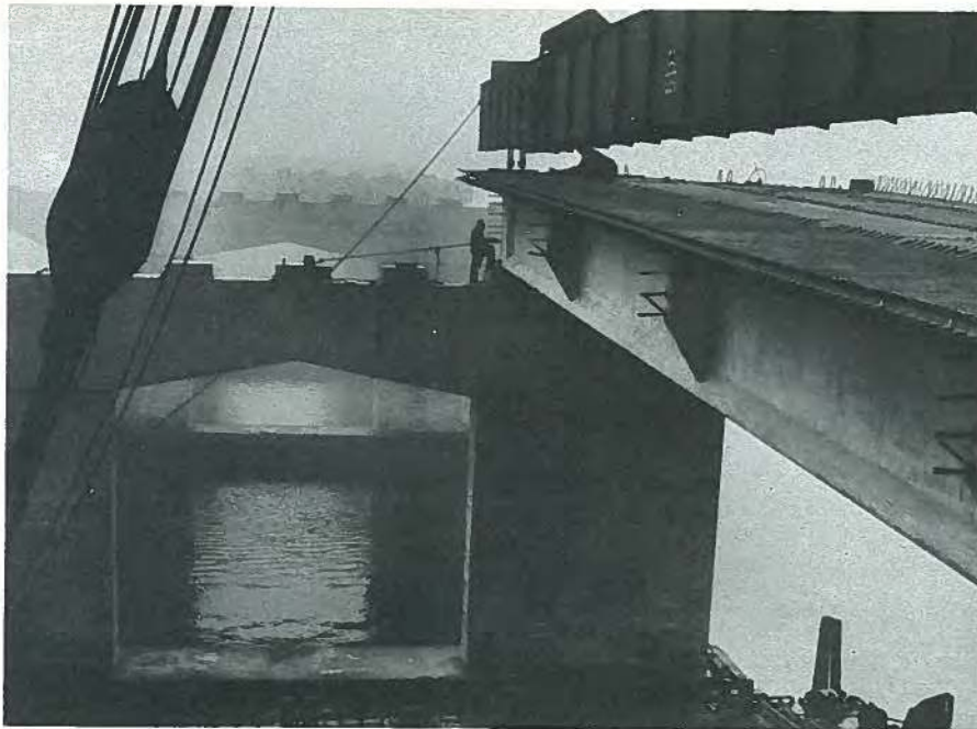
Fig. 8. Erection of 135-ft long precast prestressed concrete girders barged from Cape Charles, Virginia to Long Island, New York, a distance of about 350 miles, for the Cross Bay Boulevard Bridge Jamaica Bay, N.Y. Crossing. Owner, Triborough Bridge and Tunnel Authority.
