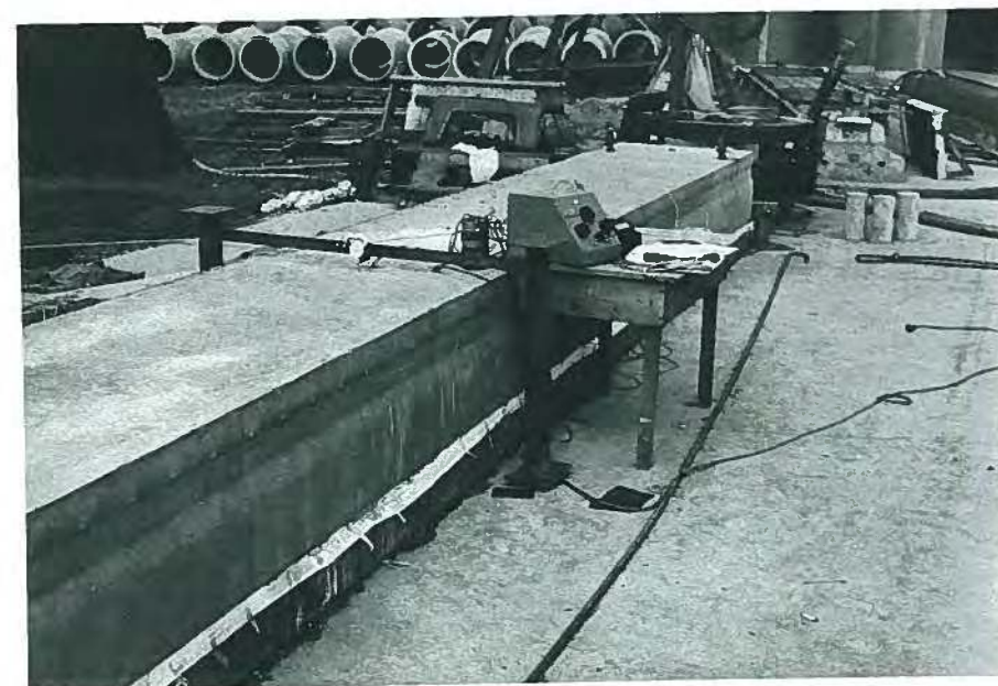
Fig. 21. Strainmeter setup for measuring strains during prestressing operation.
