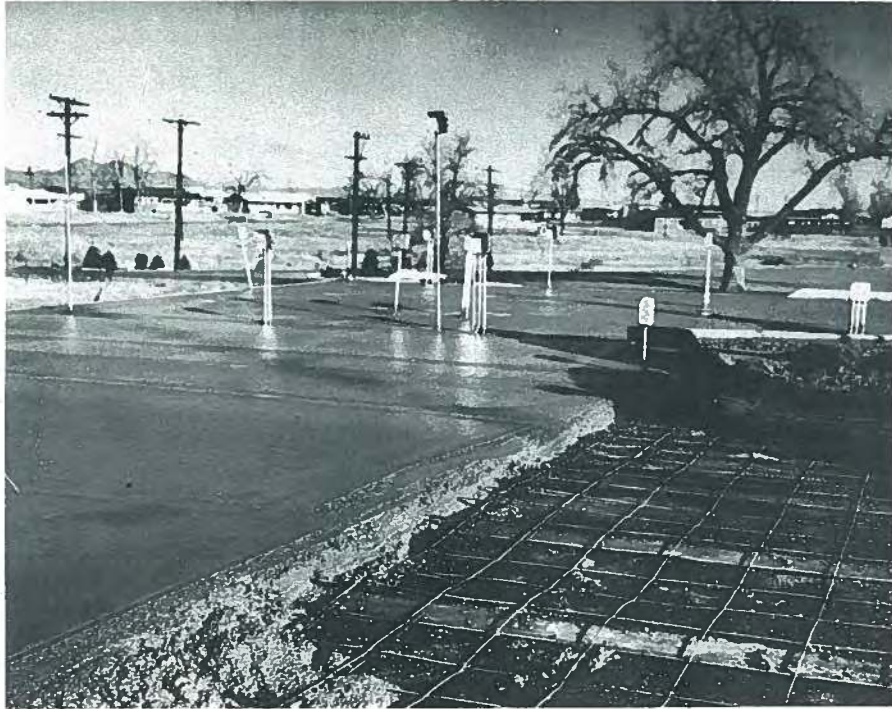
Fig. 27. In the final operation, concrete is placed and finished over the form board covering the Quadeck.
