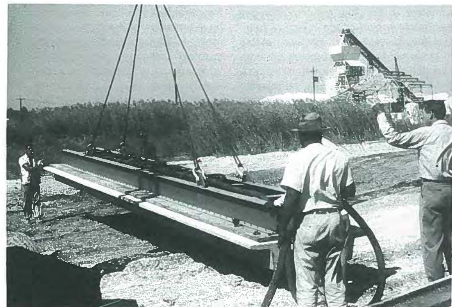
Fig. 14. Vacuum lifter in action raises and removes precast non-prestressed channel seats from the molds for later use in Loyola University's stadium. This structure is an early example of the combined use of prestressing with precasting techniques.
