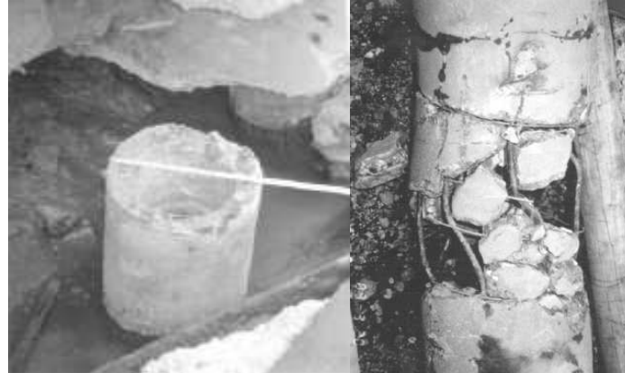
Figure 1.3 Shearing (left) and damage (right) to pile by ground displacement in Kobe 1995 and Niigata 1964 earthquakes, respectively (Finn & Fujita [2])
