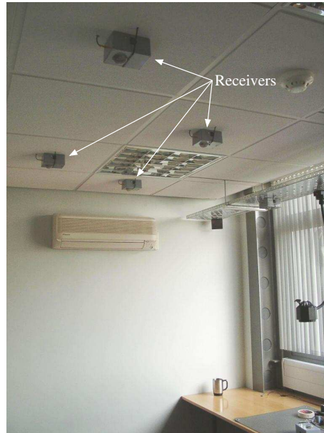
Fig. 7. Room with prototype broadband ultrasonic location system installed
