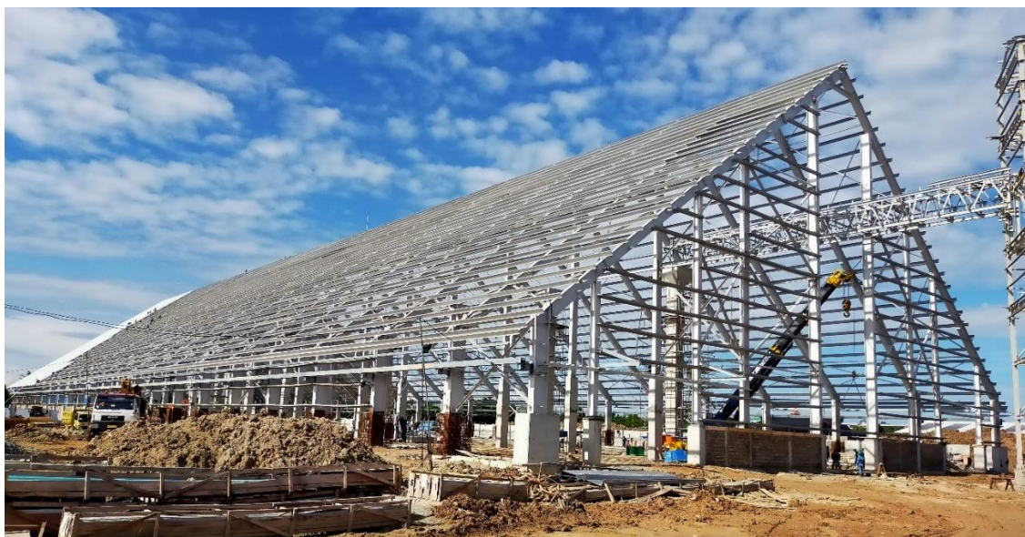
Figure 11. Installation of the GFRP Z beam purlin in a new fertiliser warehouse building.
