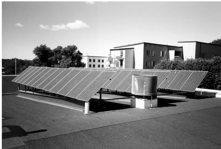
Figure 1. The Sankt Jörgen photovoltaic power plant.
