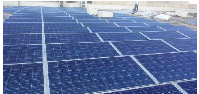
Fig. 1. Rooftop mounted Solar panels on top of the engineering building.
