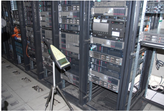
Fig 6. Measurement by 2260 Investigator in IRIB data centre server room
