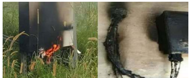
FIGURE 7. Damaged combiner box by fire [28].
