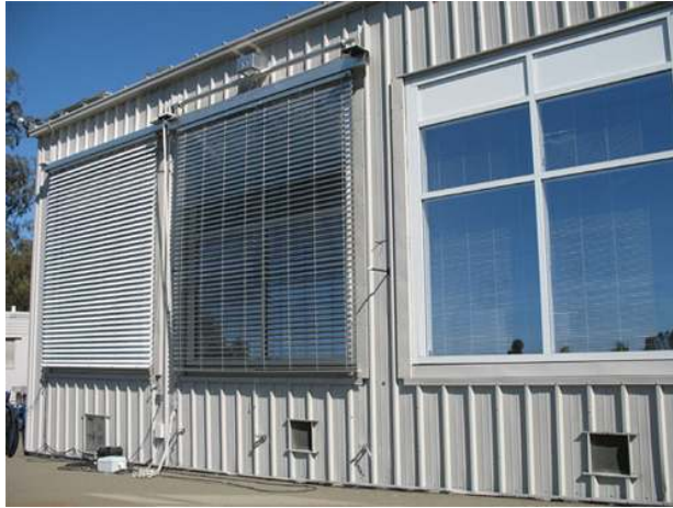
Figure 10. Exterior and interior Venetian blind systems Source: LBNL
