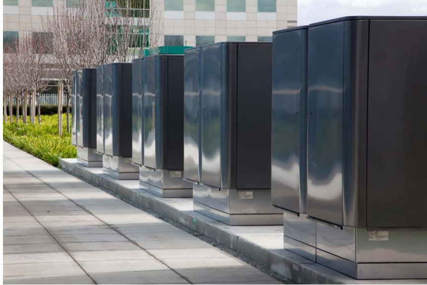
Figure 20. Bloom Energy fuel-cell power system
