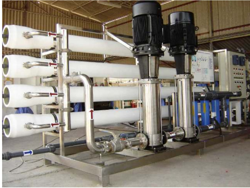
Figure 36. Reverse osmosis equipment at an industrial facility
