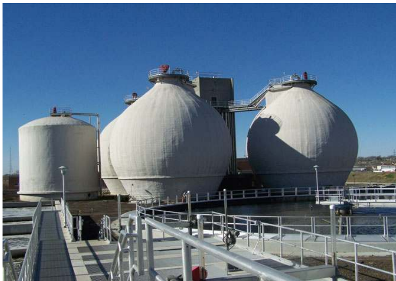
Figure 38. Anaerobic digesters at a wastewater treatment facility
