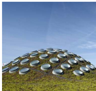
Figure 11. Green roof and skylights provide natural ventilation Source: California Academy of Sciences
