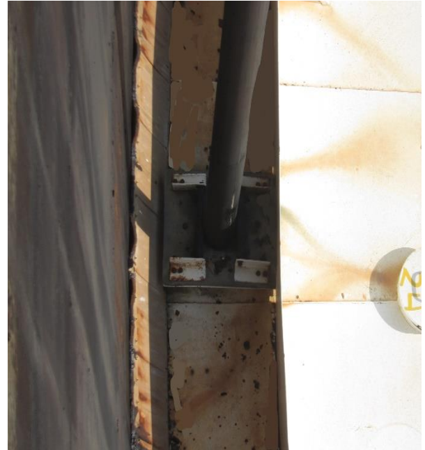
Fig. 11: Foam Blockage by Guide Pole Due to Poor Design of Foam Dam
