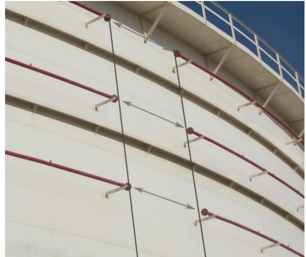
Fig. 30: Dry Strip Due to Inadequate Nozzle Separation Distance
