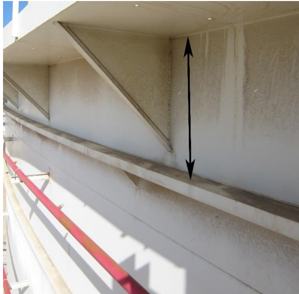
Fig. 28: Providing No Cooling Ring above Wind girder
