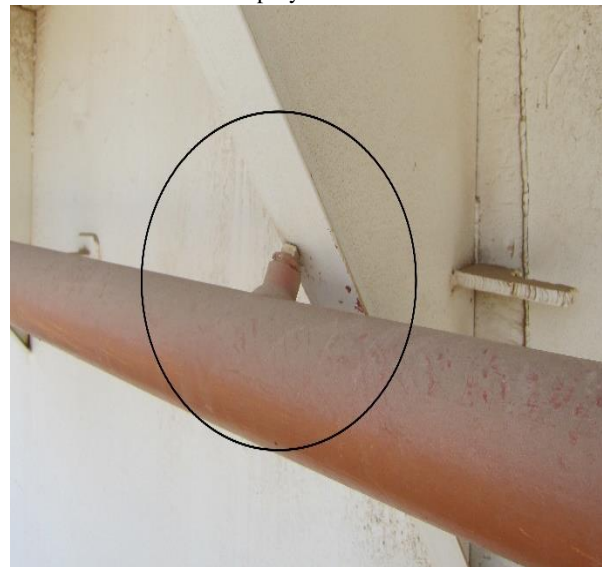
Fig. 27: Blockage of Outlets by Tank Appurtenances
