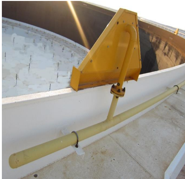
Fig. 53: Foam Solution Ring Main Above Walkway
