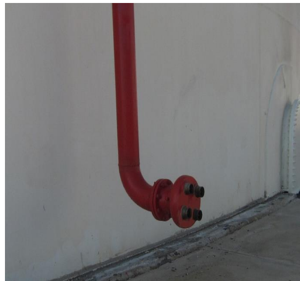
Fig. 21: Piping Terminated at Tank Bottom
