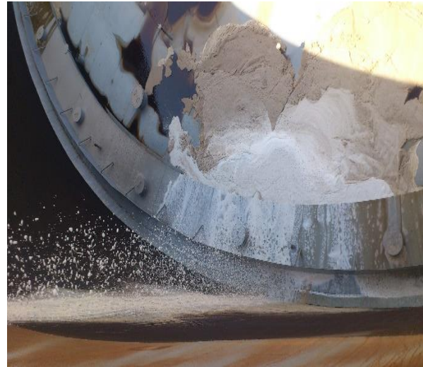
Fig.3: Excessive Foam Drainage from Foam Dam Causes Localized Foam Application
