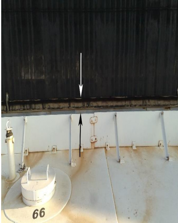
Fig. 9: Inappropriate Foam Dam Height
