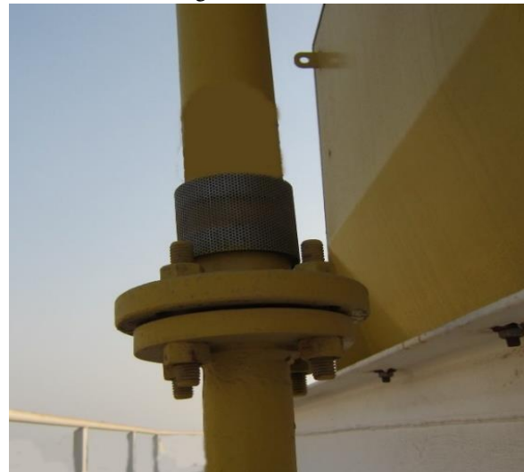
Fig. 55: Incompatible Ring Main Branch Pipe and Foam Pourer Flange Sizes
