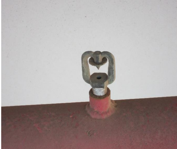
Fig. 23: Inappropriate Spray Nozzle - Full Cone Medium Velocity Nozzle
