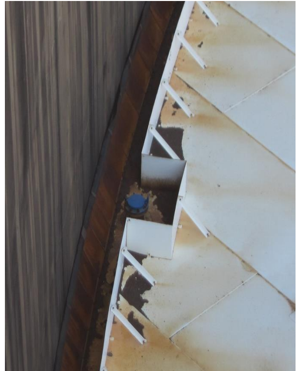
Fig. 7: Tank Components Included in Dammed Area
