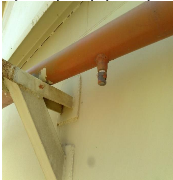
Fig. 29: Water Spray Nozzles Installed in 6 O'clock Position of Ring Main
