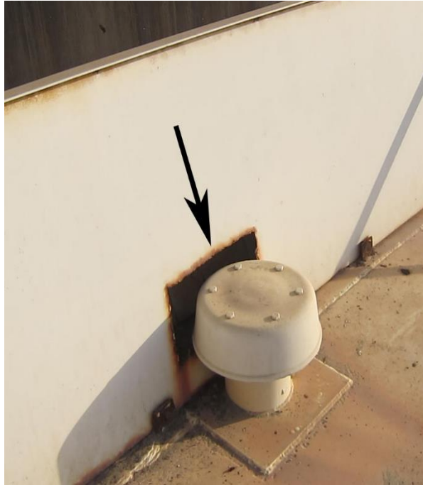
Fig. 5: Detrimental Foam Dam Modifications
