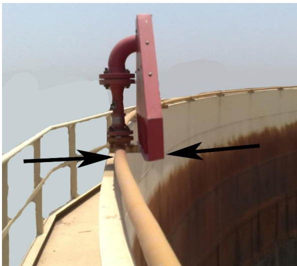
Fig. 49: Foam Pouwer Sticking inside the Tank
