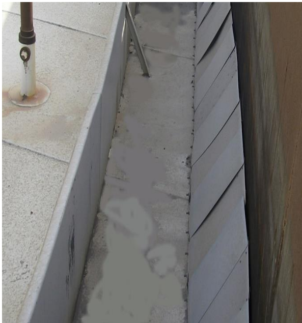
Fig. 10: Inappropriate Foam Dam Width
