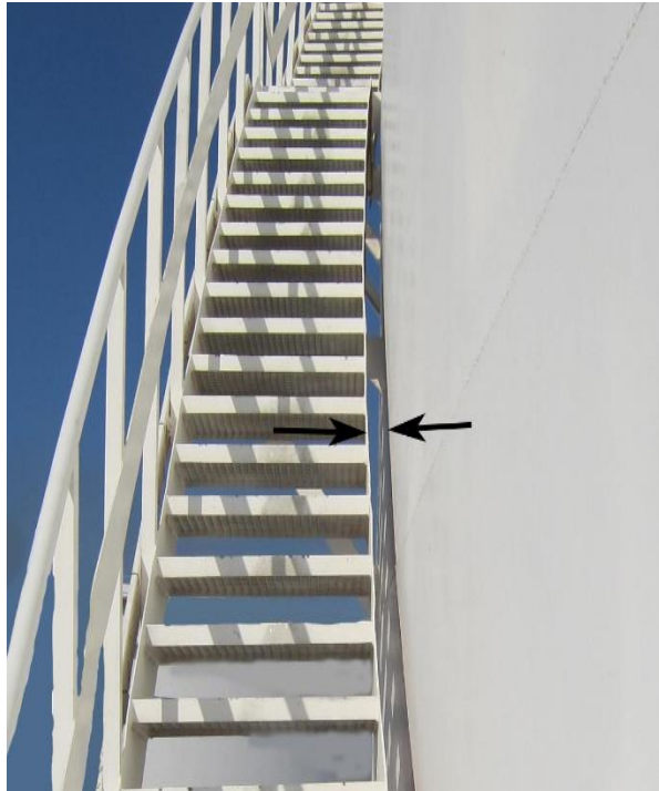
Fig. 20: Spiral Stairway Separated from Tank Shell
