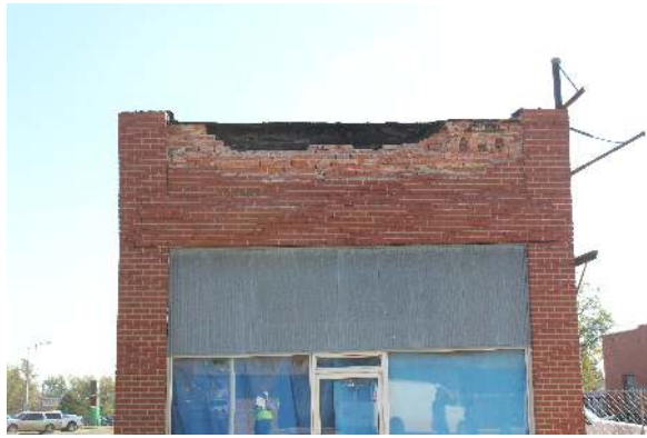
(a) Parapet wall inertial failure, Kaikoura earthquake (EERI, 2018)
