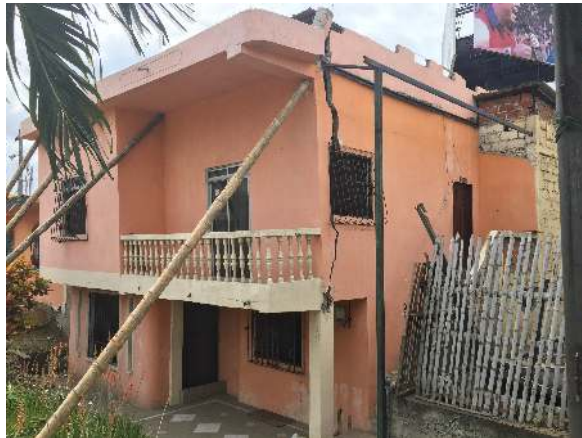
(e) Muisne earthquake inter-storey drift failure, Ecuador (EERI, 2018)
