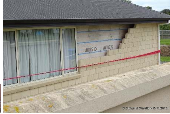
(b) Façade masonry wall inertial failure, Kaikoura earthquake (EERI, 2018)
