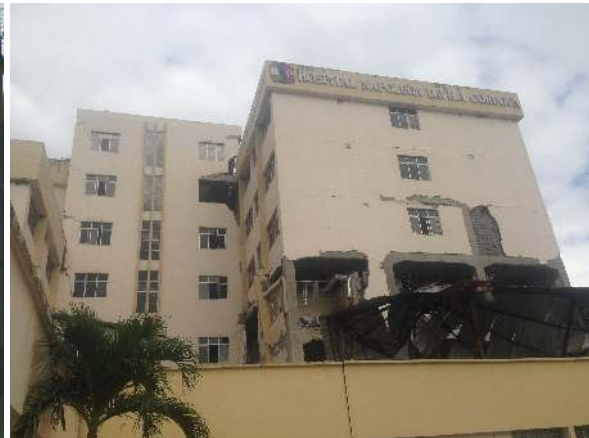
(f) Muisne earthquake mix of inter-storey drift and inertial failure, Ecuador (EERI, 2018)
