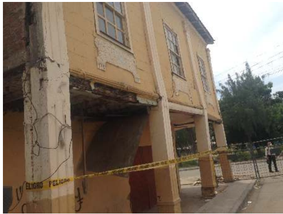
(c) Muisne earthquake inter-storey drift failure, Ecuador (EERI, 2018)
