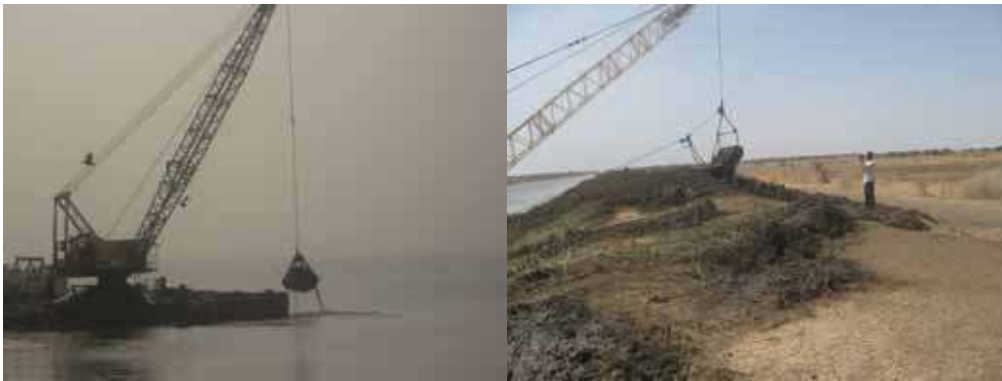
FIGURE 24. Dredging in Roseires Reservoir and an irrigation canal in Sudan ( photo credit: Seleshi B. Awulachew ).
