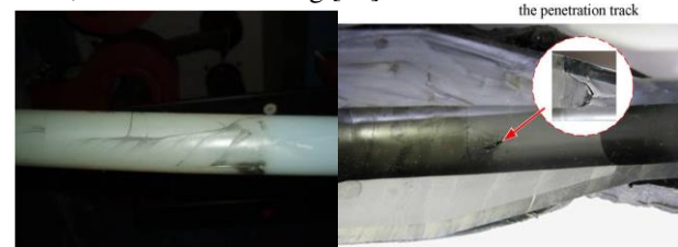
Figure 7. carbonization inside the cable termination (left) [28], penetration track on the cable joint (right) [29].
