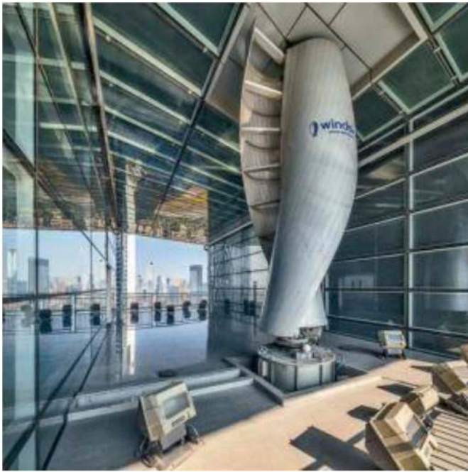
Fig. 9. A wind turbine installed in the Pearl River Tower building (Source: SOM, Pearl River Tower, Jan 2014. www.SOM.com ).
