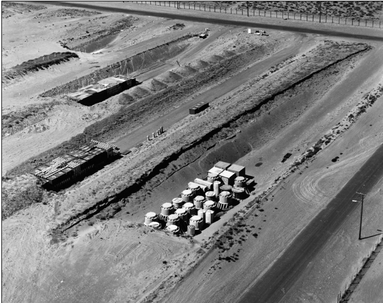
Solid Waste Burial. This photograph shows an open trench receiving solid waste in the 200 West Area burial grounds. Afterwards, burial grounds are covered with soil.
