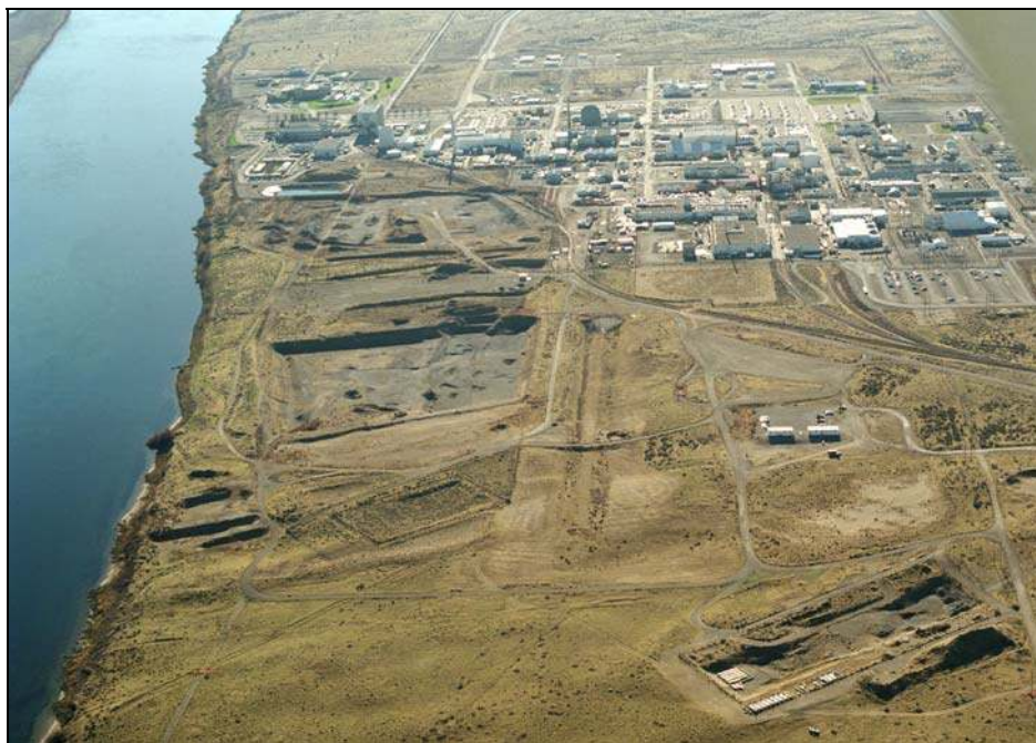
Figure 6.9. Aerial Photograph of 300-FF-5 Looking South with the Columbia River on the Left. The North and South Process Ponds (center-left) are partially excavated.
