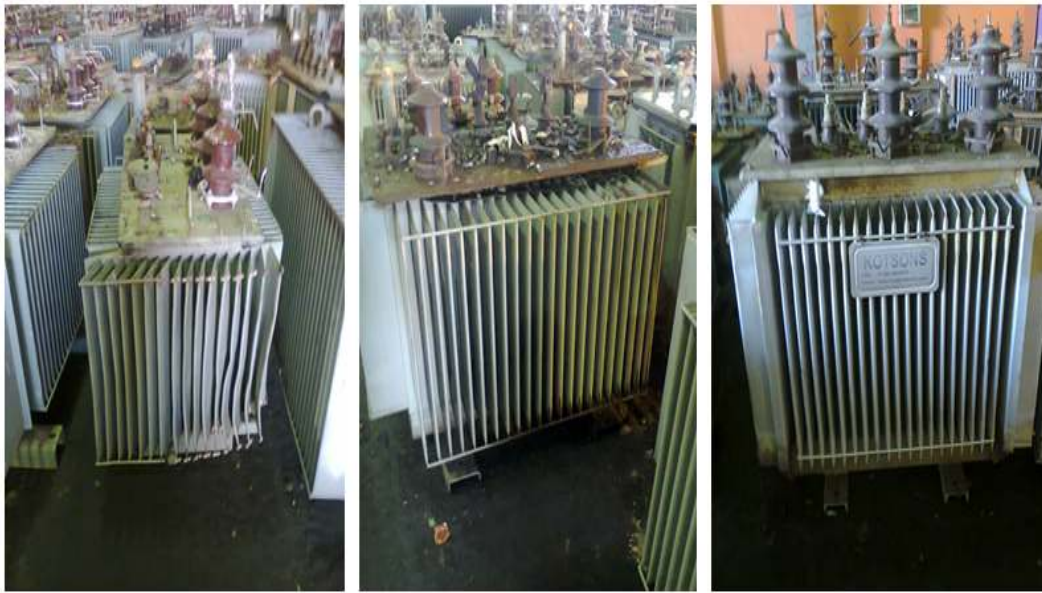
Fig. 9: Faulty DT samples from Baghdad electrical grid maintenance site as follows: pivot damage, oil leaks, and shorted winding.
