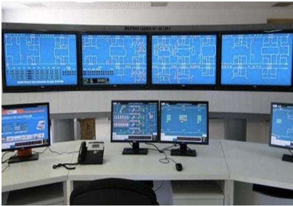
Figure 12. Example of control center operation for O&G industry [241]
