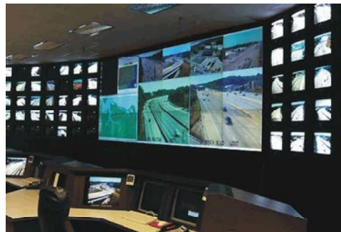
Fig. 3: Traffic Management System
