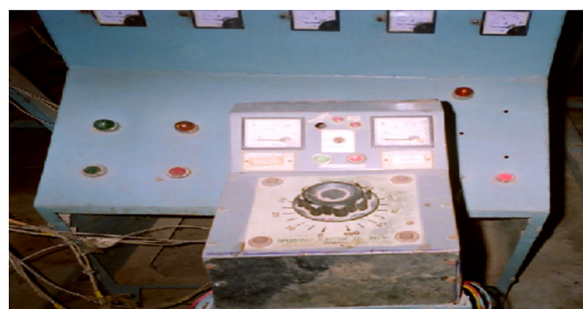
Fig. 4 Dimmer speed regulator
