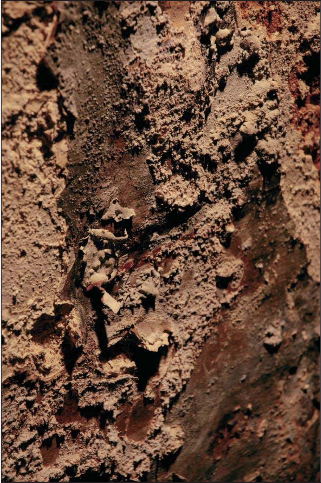
Figure 66: Detail (A8-8) Image of surface conditions: blistering, flaking, and salts (Source: C. Silva, 2006)
