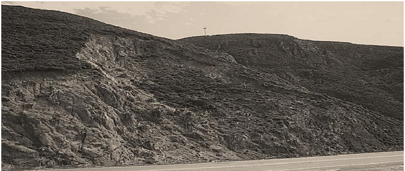
Fig.2.2 Circular failure in highly weathered, granitic rock (on Highway 1, near Devil's Slide, Pacifica, California). (Source: Rock slope engineering, 4 th edition by Duncan C. Wyllie and Christopher W. Mah.)
