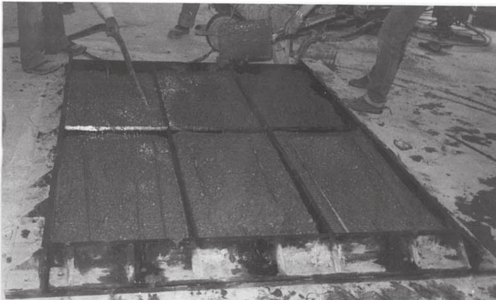
Plate 6.2 Concrete is Being Placed in the Mould and Vibrating Poker is Used for Compaction
