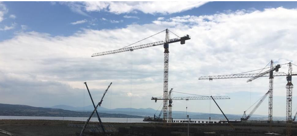
Photo 2. Piling of poles for a suspension bridge legs in the Strait of Canakkale (original)
