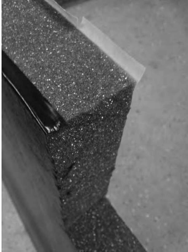
Figure 4.4.: The absorption material installed on the power pack encapsulation
