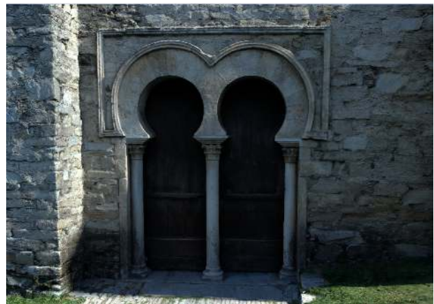
Figure 15: One of the original photographs (up) of the door of Santiago de Peñalba, Leon, Spain and an synthetic view (down) of the 3D model with acquired appearance, rendered using physically based methods for a different viewpoint and illumination.
