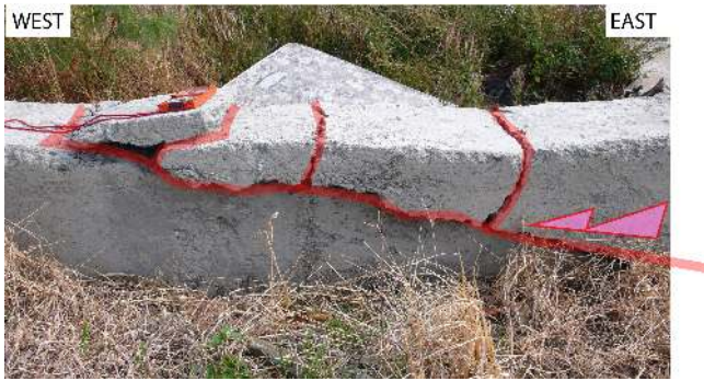
Figure 6. Field photograph of compressive features affecting recent concrete dykes after the Hengchun earthquake (26 December 2006, M_L = 7.0 ); see location in Fig. 1 near the Fang-Shan village ( 22.26^\circ N, 120.66^\circ E). The red compass gives the scale of the outcropping deformation (20 cm). The thrust is associated with three back thrusts, highlighting a small pop-up (below the compass). The red arrow reveals the thrusting component that affects the new concrete dykes.
