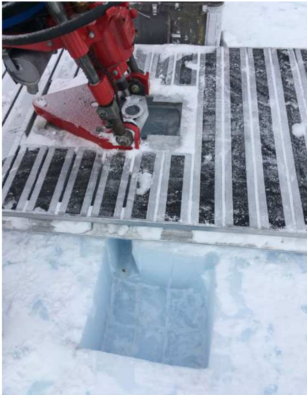
Fig. 6. An ice sump was cut into the surface of the blue ice to collect the fluid and chips as they were pumped to the surface.
