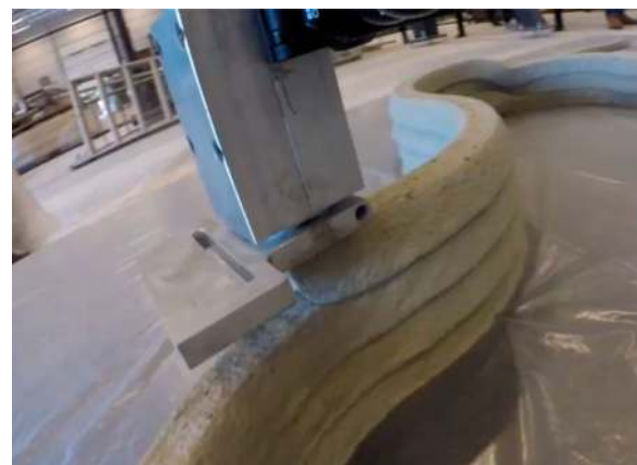
Figure 6. 3D concrete printer in operation. No-slump concrete leaves the nozzle as a relatively stiff continuous filament.
