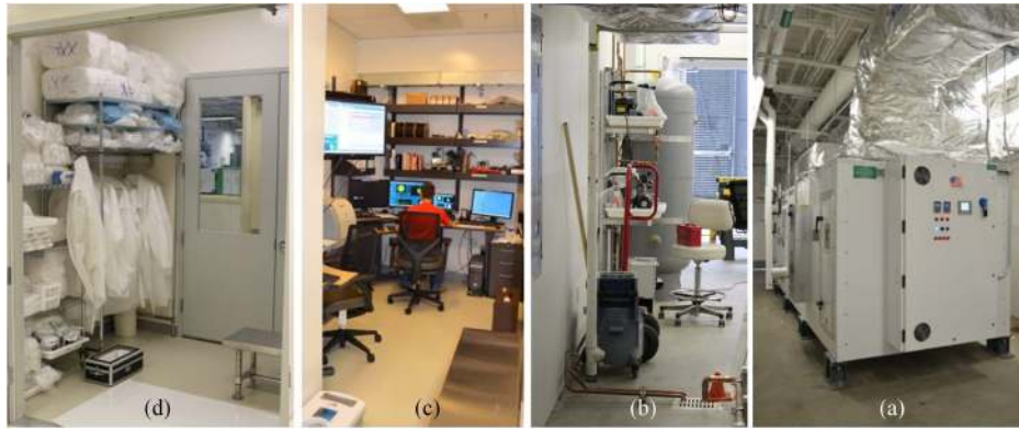
Fig. 2 XROL at the ALS: mechanical room with (a) air conditioning system and (b) air compressors, air dryer, and a 200-l reservoir tank; (c) control room; and (d) gowning room.
