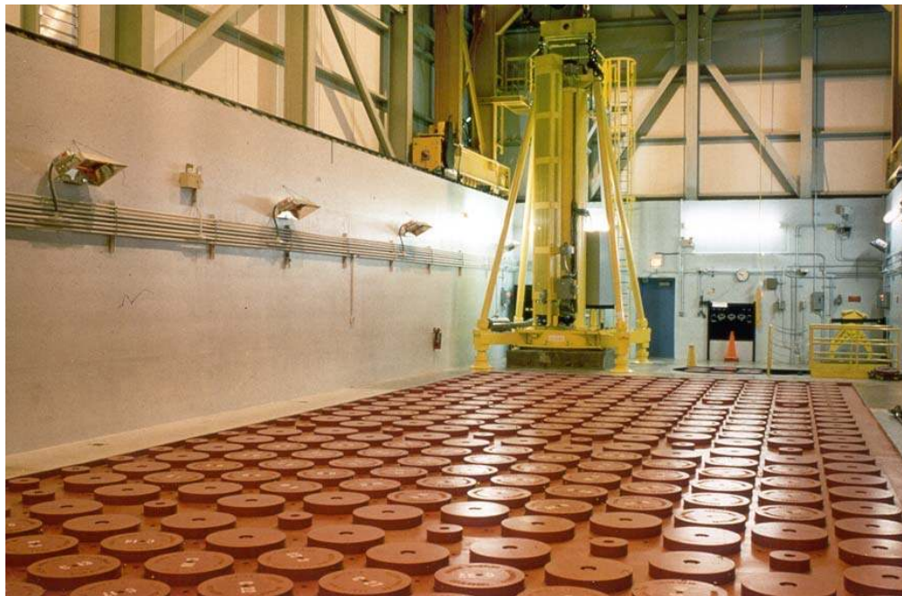
Figure A-5. Fort St. Vrain modular vault dry store (MVDS) showing charge face.
