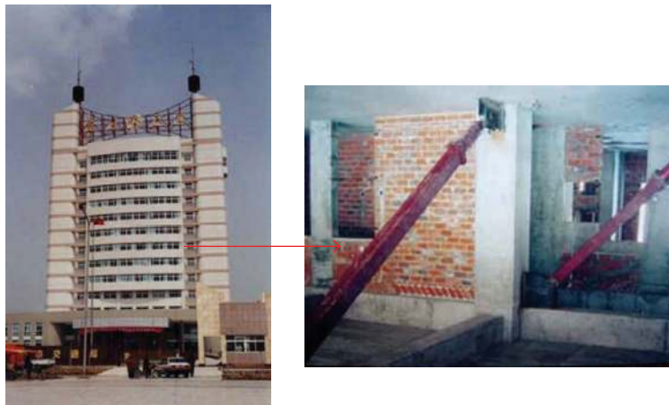
Figure 9: Viscoelastic dampers in Suqian Communication Building.
