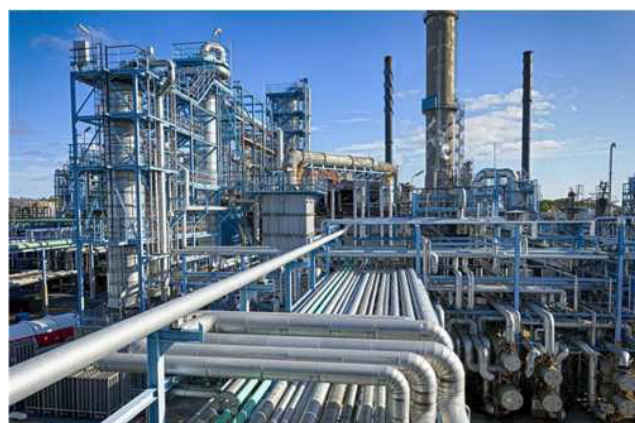
FIGURE 2. Illustrative industrial scenario with several arrays of pipe structures.
