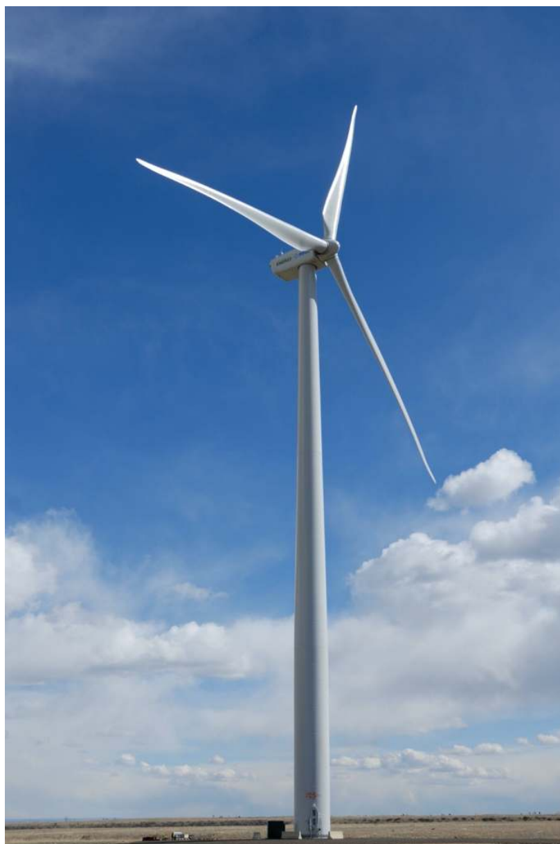
Figure 5. DOE-owned 1.5-MW wind turbine located at site 4.0 at the FC. Photo credit: Jeroen van Dam, NREL
